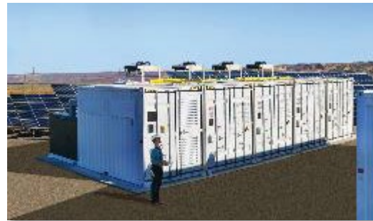
Horn Rapids Solar, Storage & Training Project
