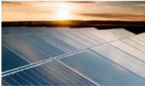
White Bluffs Solar Station (38 KWe)
